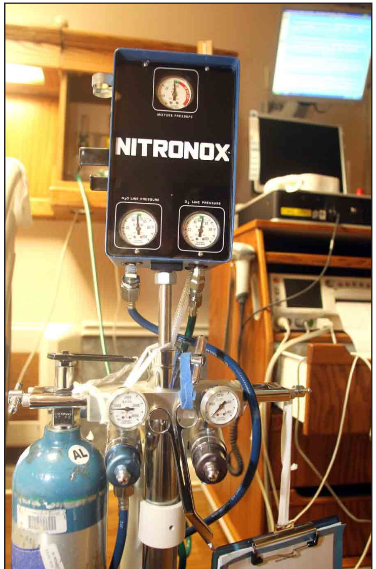
Older generation of Nitronox machine.
