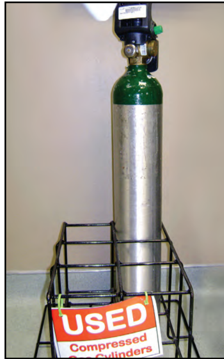
The medical gas cylinders need to be secured with an appropriate chain or stored securely in an approved holder. The storage racks also need to be labeled to clearly identify full cylinders from empty cylinders.
