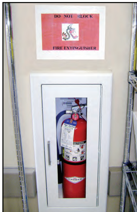
There must be clear access to the fire extinguisher.
